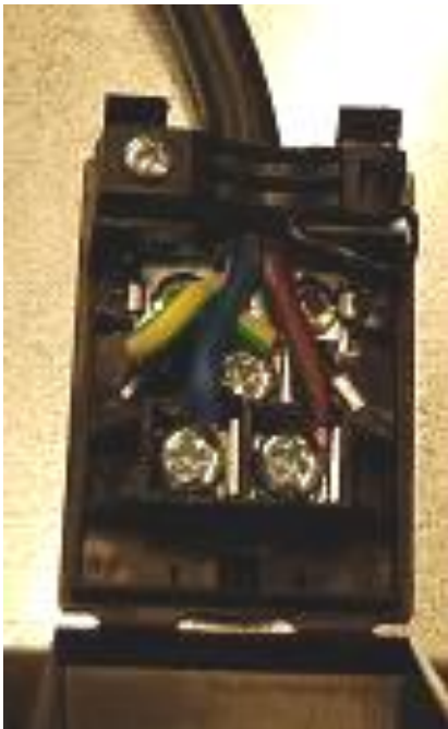
PI29.....; connection box open
