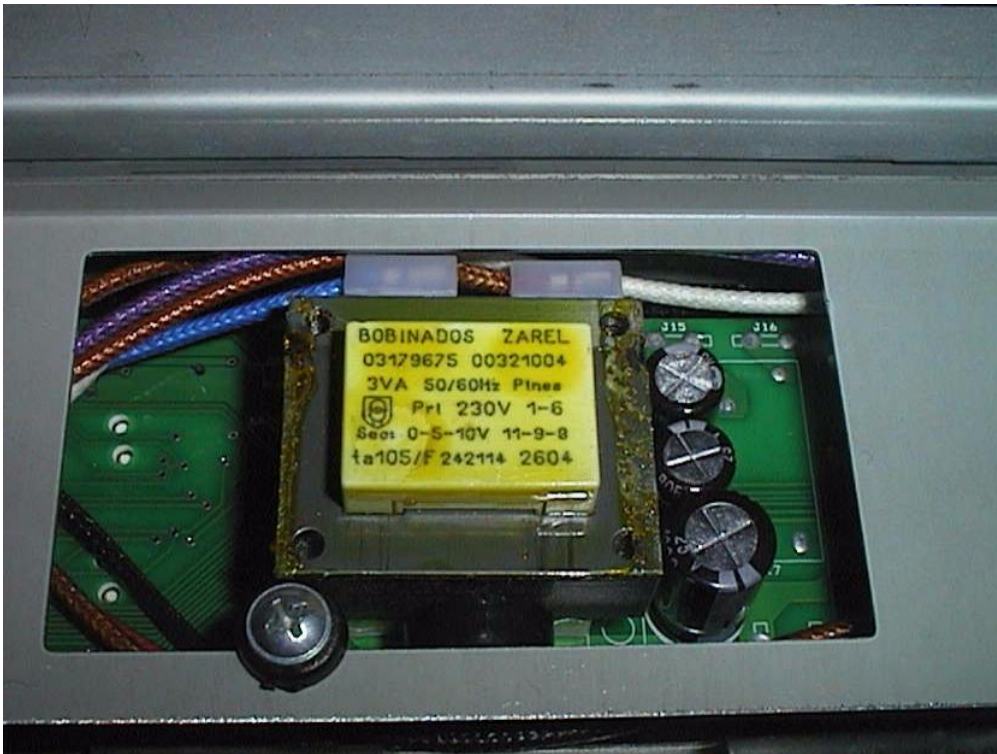
Transformer on EKA touch-control
